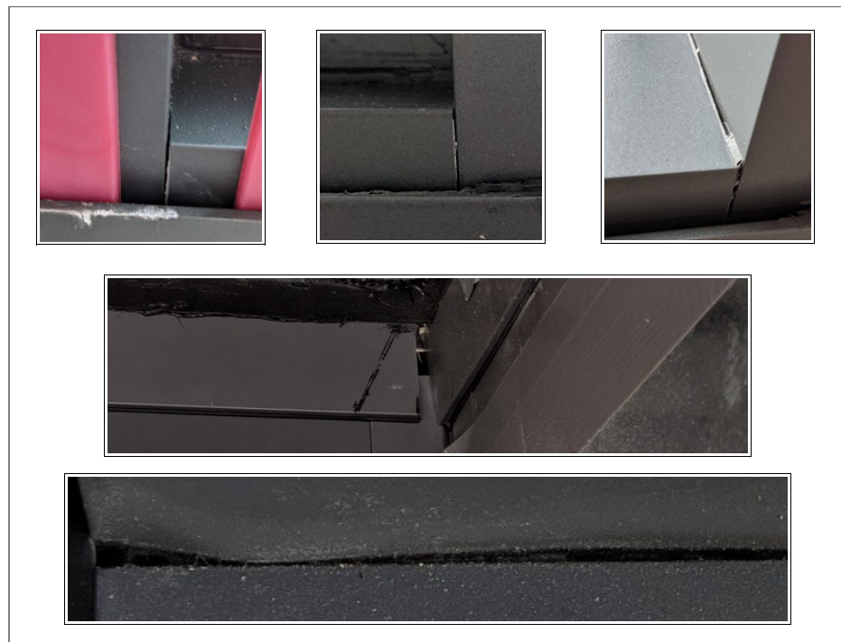
Fig. 06: Frame Joinery & Head Drive Voids that May Allow Air Infiltration
