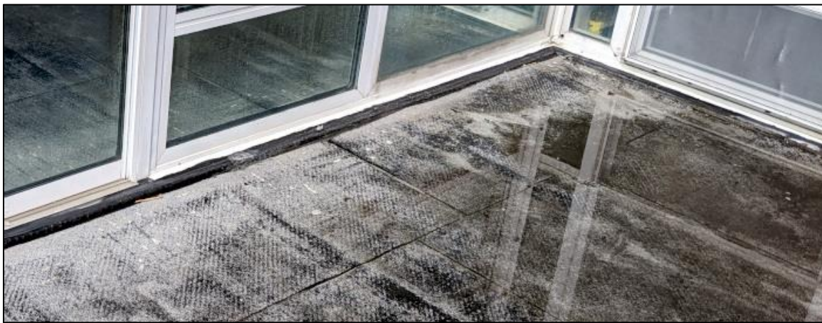
Targeted testing of plausible sources near the reported leak did not reproduce the interior leakage
